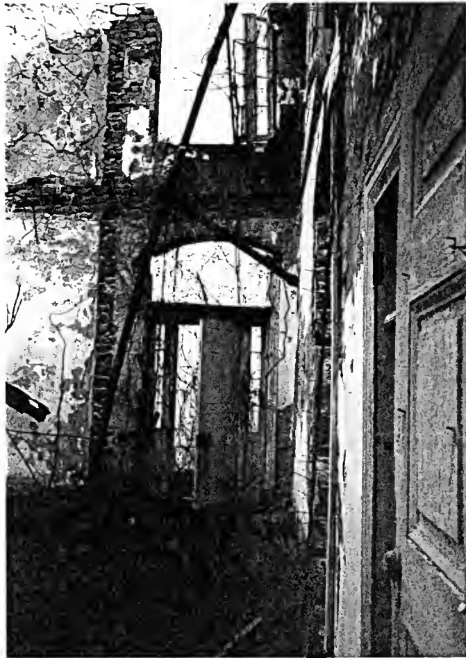
Figure 23: Second story plumbing for bathroom above central hall, leaning towards interior wall
